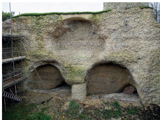
FIGURE 3: Interior of the west wall of the keep, before completion of the restoration. A pier of masonry has been inserted between the two arched recesses where the wall had been undermined, and a concrete lintel over the top of the first-floor fireplace
