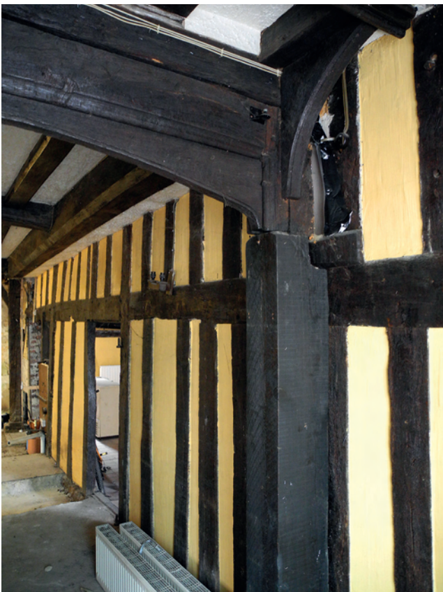
FIGURE 6: South wall of the north cross-wing (painted yellow) and the gateway into the cross-passage
