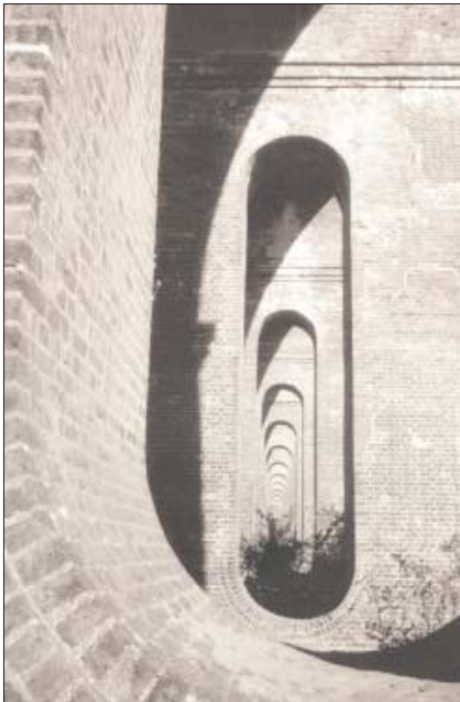
Figs 1 & 2 (opposite). Chappel Viaduct arches from the east. Centred at TL897284. Built 1847-9. Designed by the civil engineer Peter Bruff and reputed to contain 7,000,000 locally-manufactured bricks.
