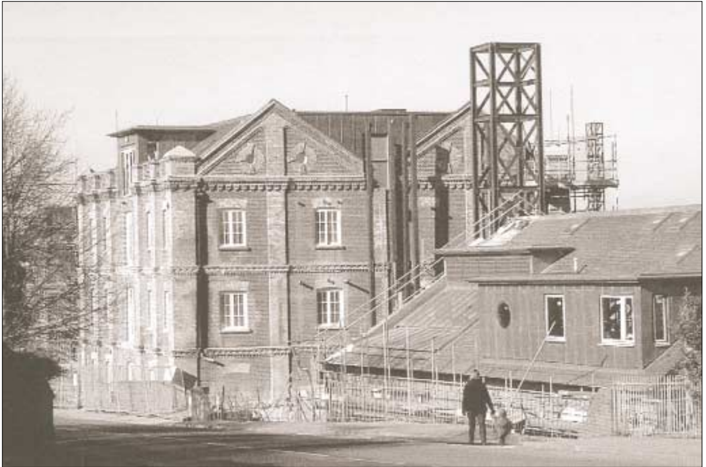
Fig 3. Mistley Maltings Number 1, constructed by Free, Rodwell & Co in 1896/7 and incorporating major technical innovations. Currently undergoing conversion into residential accommodation.
