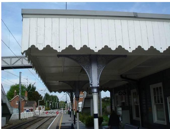
Detail of the canopy valencing and the cast-iron support columns and brackets on the up platform. The columns and brackets are of the same design as those at Stansted Mountfitchet.
