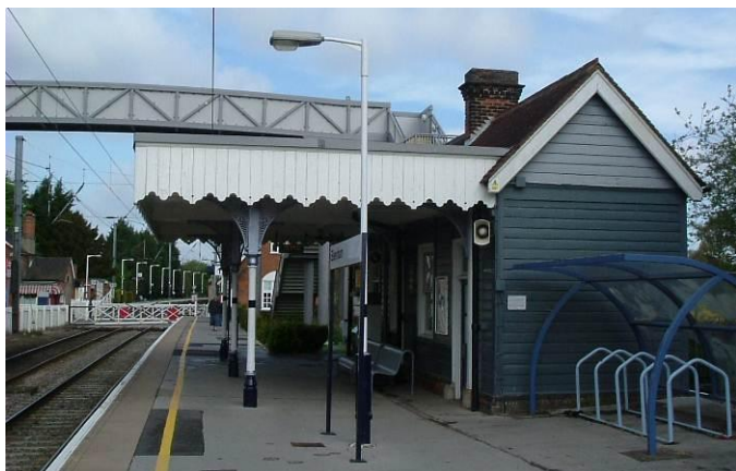
Detail of the up-side timber waiting room, Listed Grade II, with canopy valencing and supporting columns and brackets. The Station House is just on the left with the down platform beyond the level crossing.
