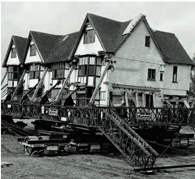
Ballington Hall in the process of being moved to its new site (April 1972). (photo: © Historic England)
