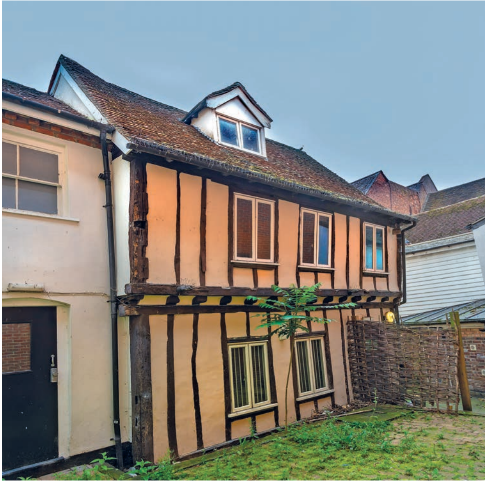
FIGURE 129: South-facing jettied side of Part D, rear of 25 Head Street (corpus no. 28). The wall studs have been largely replaced
